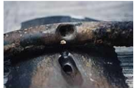
Corrosion and hole in larger gas pipe caused by smaller water pipe on top. Photo courtesy of Jose M. Maio, Electrical Research Institute, Mexico. Source: http://www.corrosion-doctors.org/Localized/sewer.htm ; accessed May 5, 2006.
